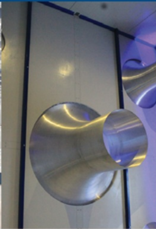
Air Flow Chamber, India.
