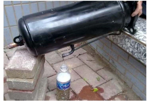
Figure 6-2.8: Draining oil from a compressor
